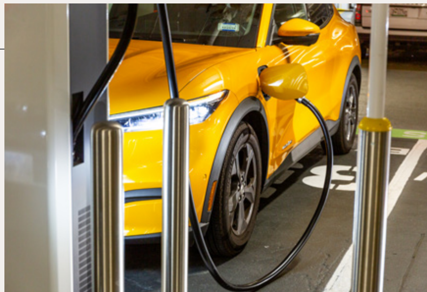
EV CHARGING AT GEORGETOWN PARK / Washington, D.C.
